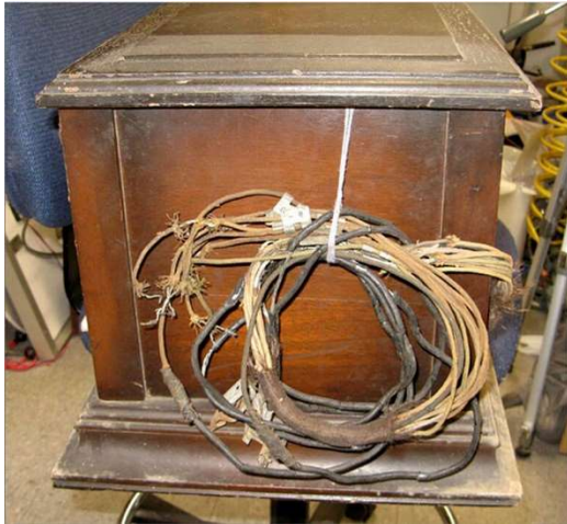
Figure 1 - Hard wired battery cable beyond salvage.
